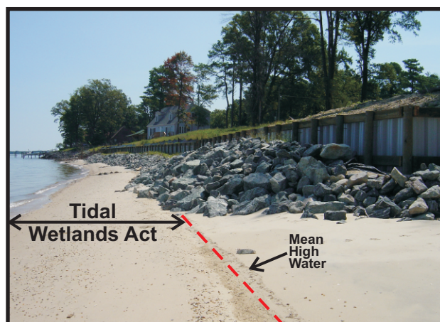
Figure 8B. A retention and bulkhead in Westmoreland County, Virginia, a non-jurisdictional locality, has impounded bank sands decreasing the amount of sand available to the beach and dune system. The mean high water line is the limit of the Tidal Wetlands Act jurisdiction.
