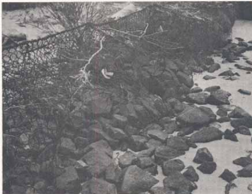
Figure A2B. West Shore Site, close-up of the structure. Note failure of wire and loss of rock.
