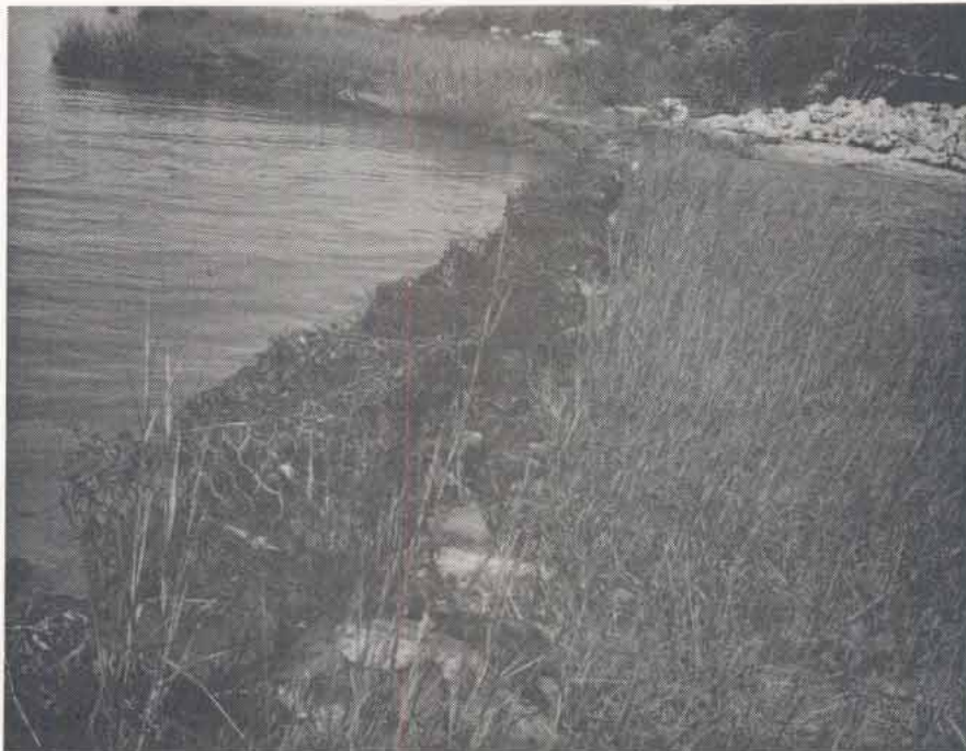
Figure A14B. D. Vann Site, closeup of north end of the structure. Basket wire deteriorated with massive failures.
