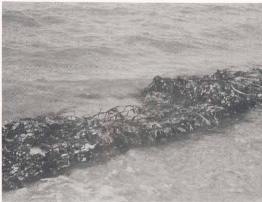
Figure AIOB. Silver Beach Site, closeup of the structure. Note the failure of wire in middle of sill.
