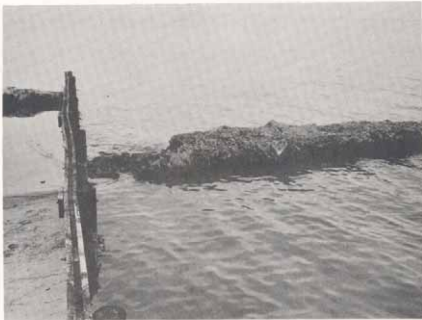
Figure A22B. Herndon Spur Site, closeup of spur. Note failure at junction point at groin.
