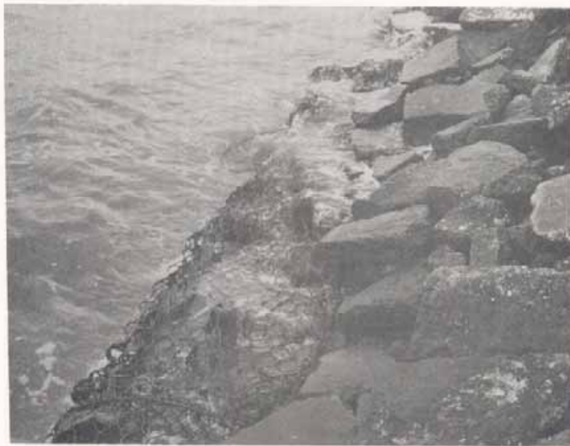
Figure AI7B. Mizelle Site, closeup of the structure. Note failure and broken concrete along top of baskets.
