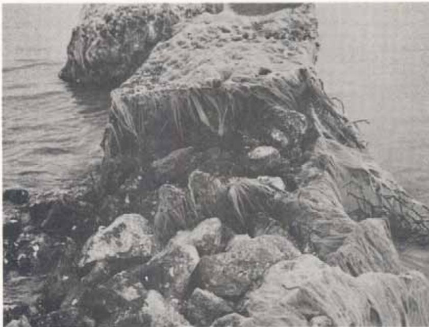
Figure AlSB. Herndon Site, closeup of sill installation 3 adjacent to the bulkhead. Note failure at junction point.
