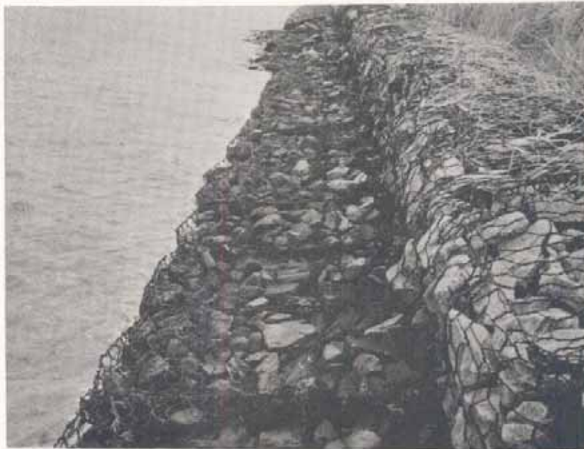
Figure A3B. Mr. Abernathy's House, closeup of the structure. Note failure of wire along top of lower gabions.
