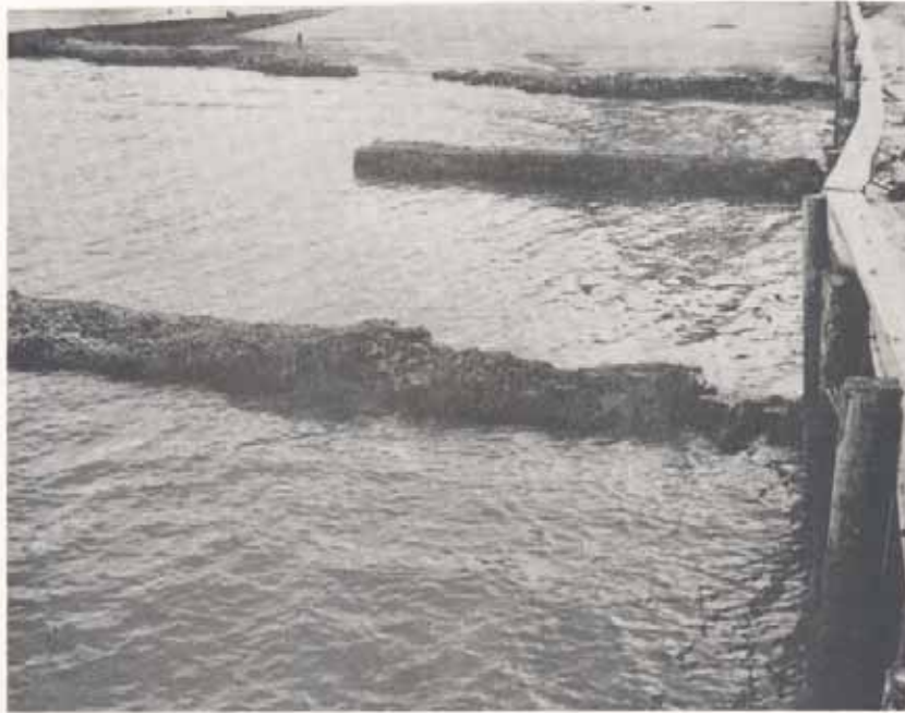
Figure A22A. Herndon Spur Site, looking west at spur and sill structures.
