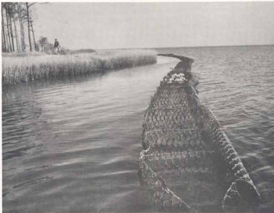
Figure AI9A. Funston Sitet looking east along the structure. Note unfilled basket, job still incomplete.
