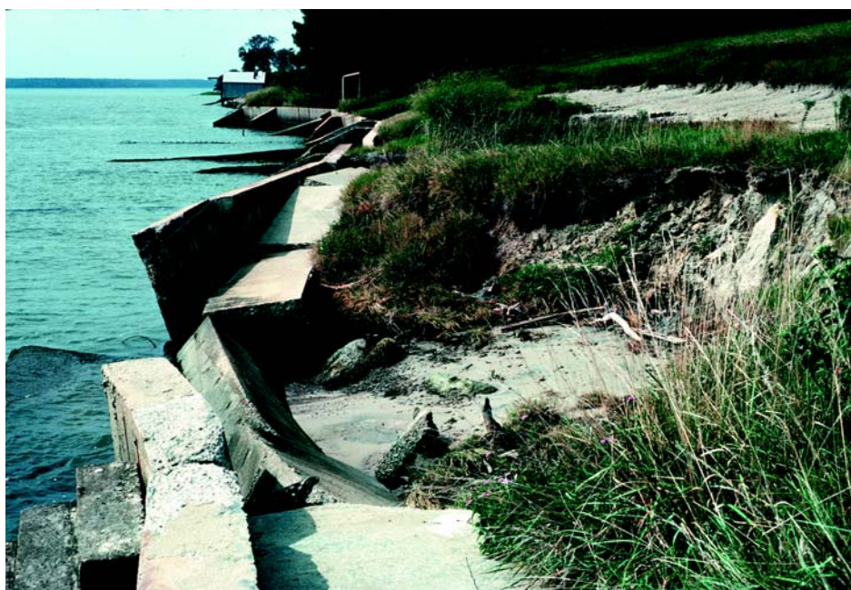
Figure 15B (bottom) Concrete seawall failure due to hydrostatic loading.
