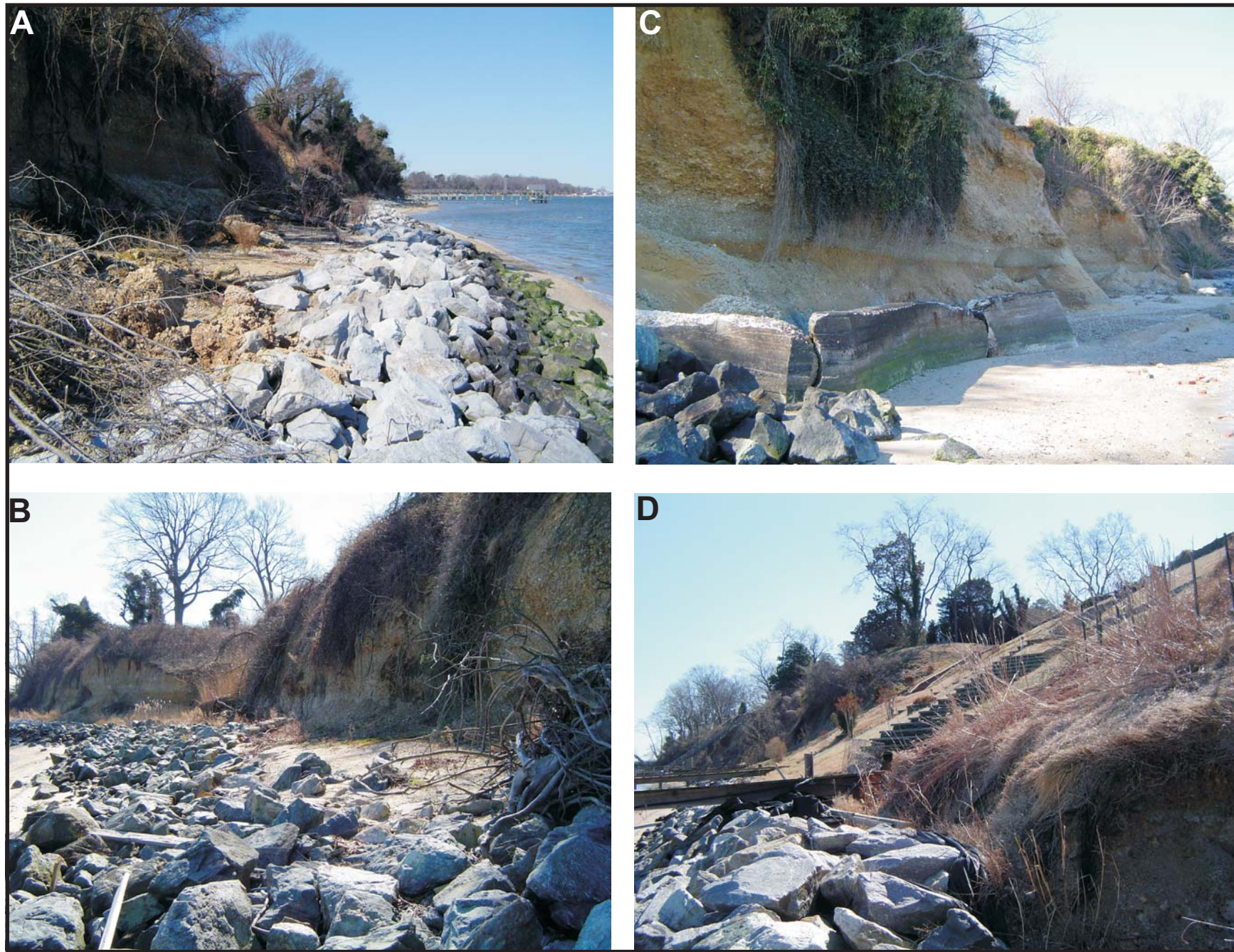
Figure 9-2. Ground photos showing the York River shoreline in the vicinity of the Moore House. Photos A and B show the rubble revetment and eroding shoreline; photo C shows the concrete structure; and D shows the grading of the shoreline on the private property near Moore House. Photos taken 3 March 2005.
