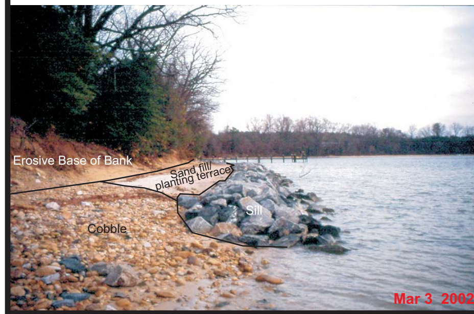
Figure 1-6 . Photos of Window 8 showing the elements of the sill project. These photos were taken before the marsh grass was planted.
