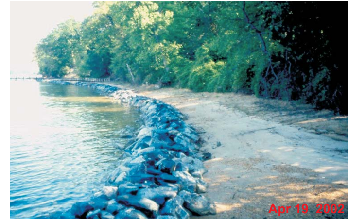
Looking north from the pier at Window 3. Spartina patens have been planted along the sand fill/terrace.
