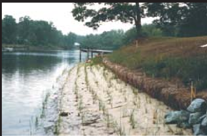
Minor bank grading and temporary toe protection utilizing straw bales was used first then Spartina alterniflora was planted to establish a marsh fringe.
