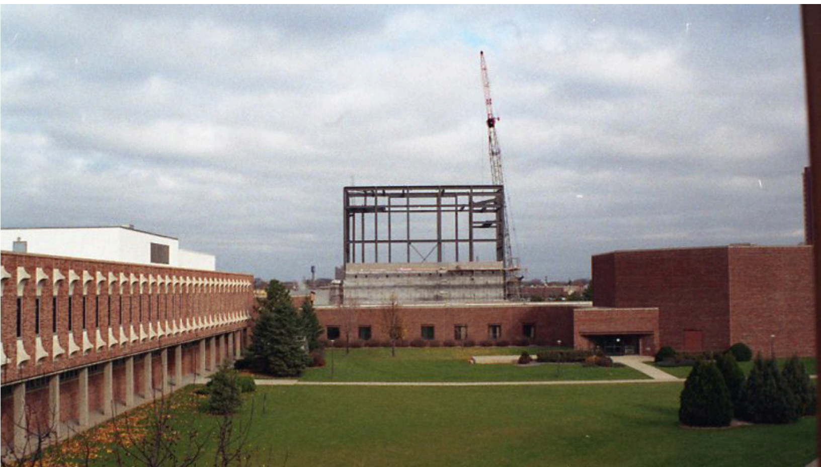
E.M. PEARSON THEATRE This image shows the new theater building under construction in 1993.
