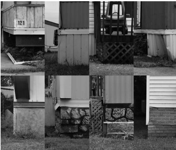
Skirting of mobile homes in various materials. [Photographs by author]
