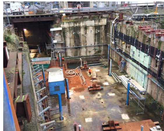
(d) Recent current situation of the defected area (Photo taken by Dipl. Ing. S. Hein – December, 2015)
