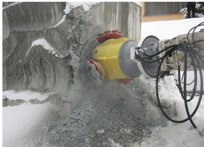
Fig. 8. A view of the KR150 roadheader arm with the new head solution with asymmetrical disc tools during one of the field tests (Gospodarczyk et. al 2010), (Kotwica et. al 2013)
