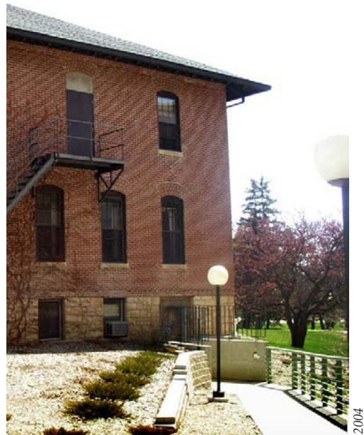
A basement-level door and access ramp were added to the west façade of MRC in 1996.
