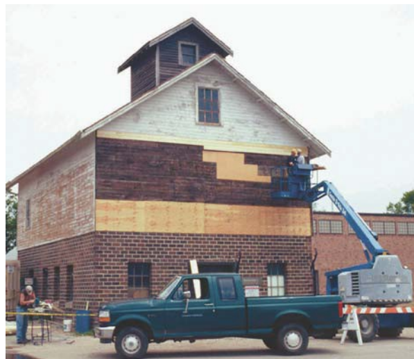
Repairing distinctive wood elements is one of the most cost-effective investments UMM can make in retaining the historic character of dormers, window muntins, and surviving WCSA buildings. Shown here: the shiplap on the Seed House is replaced with the same material and dimension in the 2003 rehabilitation.
