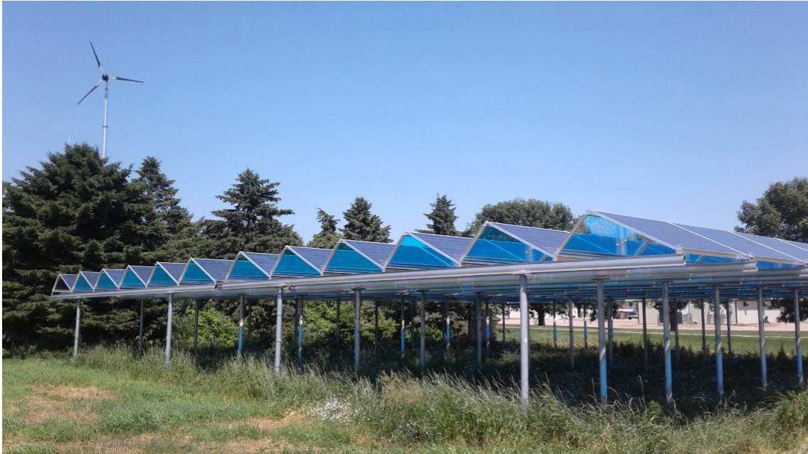
Figure 6: The 50 kW solar array installed at the WCROC dairy farm.
