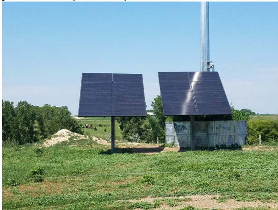
Figure 5: The 4 kW solar array installed at the WCROC dairy farm.
