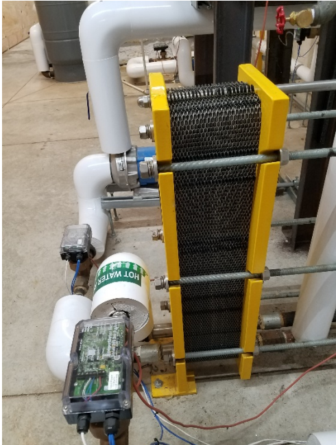
Figure 12: A plate cooler in the new utility room at WCROC.
