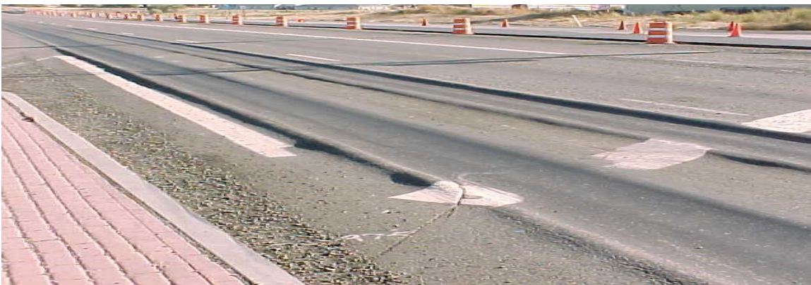
Figure 3. Rutting in Flexible Pavement (6)
