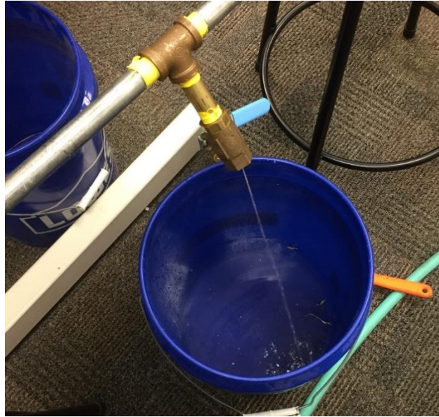
Figure 4.20. The leak created by marginally opening the middle valve
