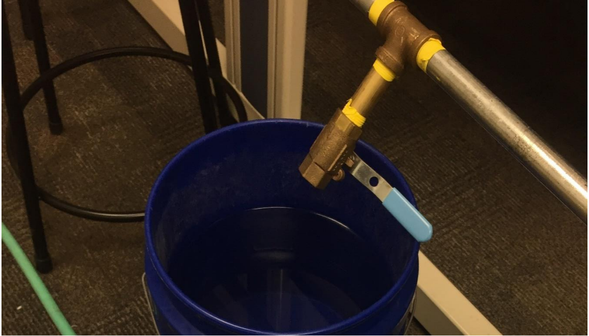
Figure 4.12. Water running at full pressure (middle valve is closed)
