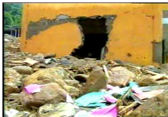
Figure 3. Effects of a debris flow on houses in Ban Ly, (Photo in 8/2004, immediately after a debris flow)
