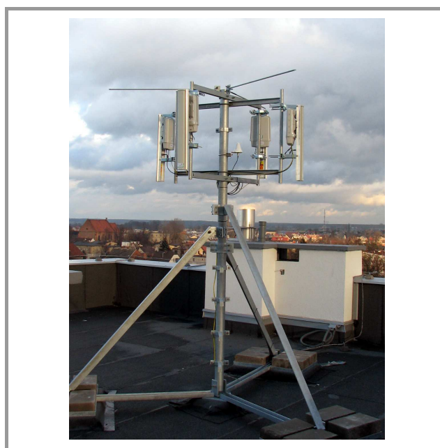
Fig. 1. One of INEA's WiMAX base station.
