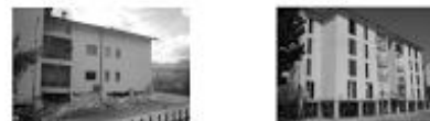
Figure 2.5. Two recent examples of severe damage attributed to the soft first story irregularity in L'Aquila earthquake, Italy in 2009. (Photos, left: Holly Razzano, Dogemiloh) and in Lorca, Spain in 2011.
