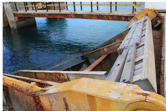
Figure 5. Major damage on movable bridge after Lua storm on March 2012.
