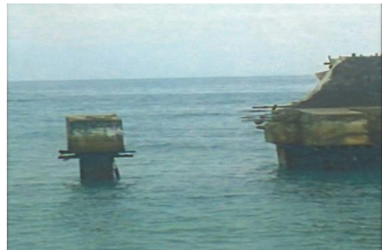
Figure 3. Significant damage of breakwater due to high wave on January 25 th , 2012
