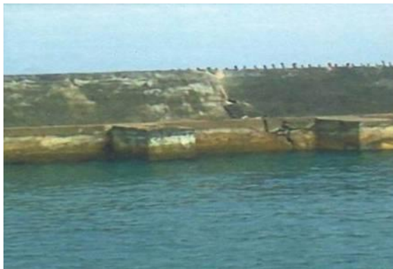
Figure 2. Cracking on breakwater concrete wall after an earthquake on January 21 st , 2012.
