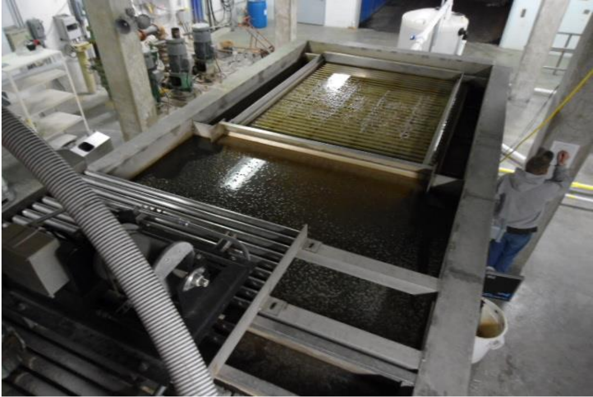
Figure 4.5.1.3. Top view of the MRI pretreatment unit.
