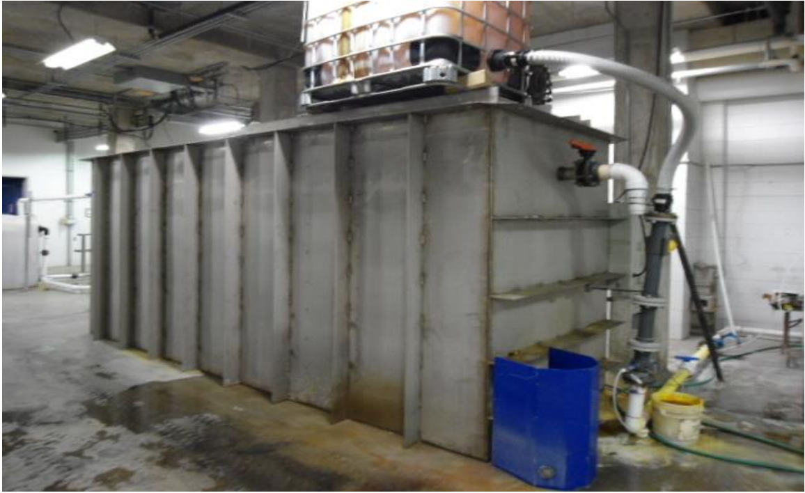
Figure 4.5.1.1. Pretreatment unit: MRI pretreatment, Raw water, acid and PACl feed point, and static mixer.
