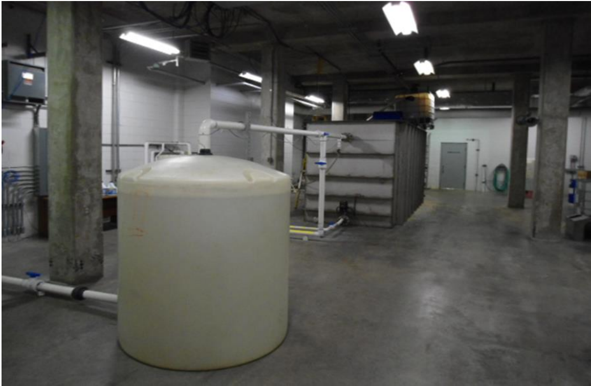
Figure 4.5.1.4. The UF feed tank and rear view of the pretreatment unit.
