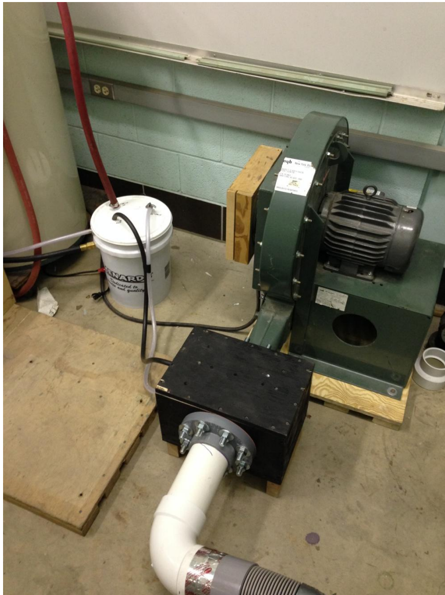
Figure 23. Small blower with new heat exchanger system.
