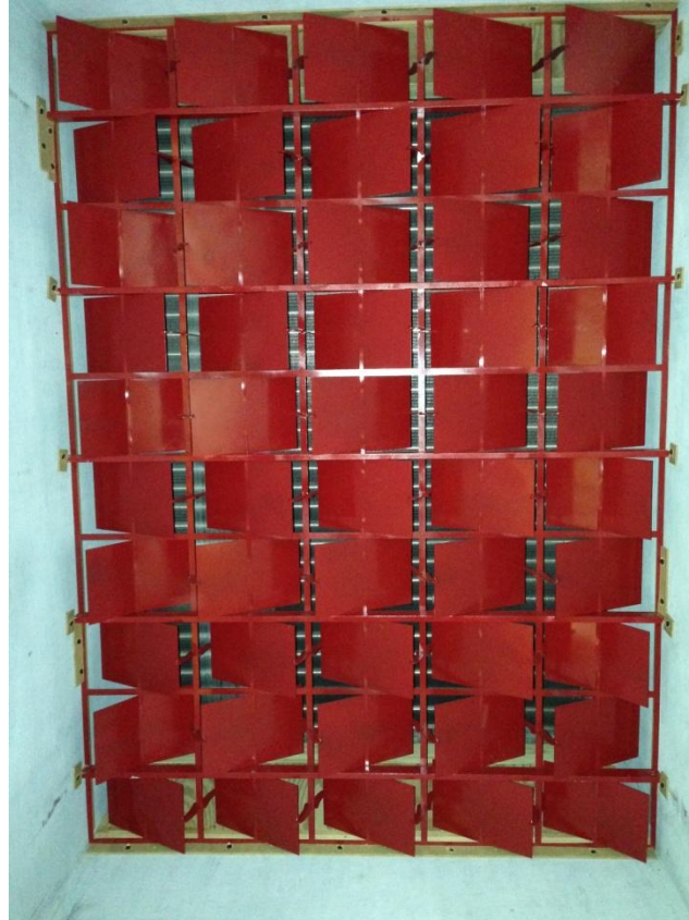
Figure 4. Flow mixer installed downstream of heat exchanger.
