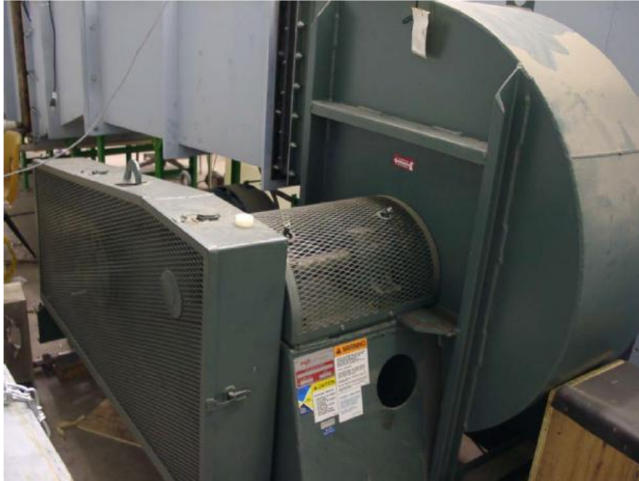
Figure 2. New York Blower used for wind tunnel [42].
