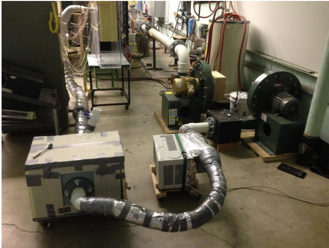
Figure 25. Entire coolant supply system.
