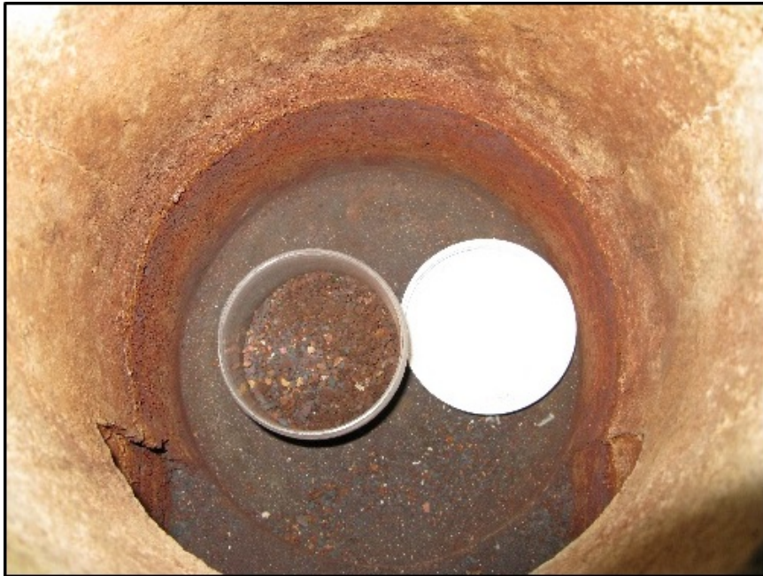
Figure 2.6: Rust removed from the bottom of the thermal oxidizer.
