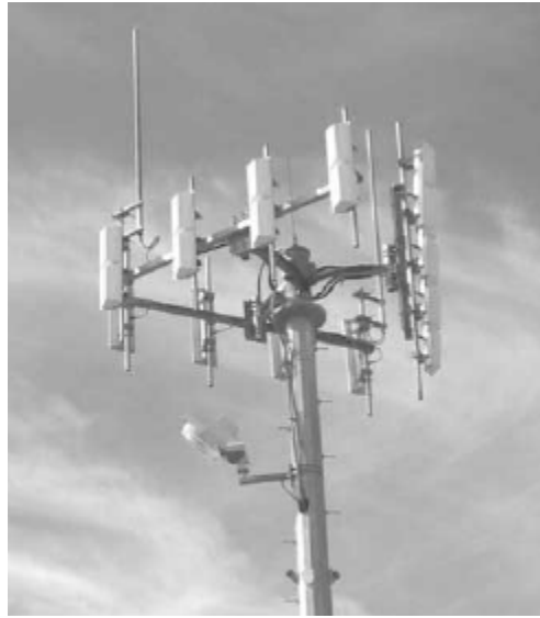
Figure 1.3: Sectorized base-station antenna
