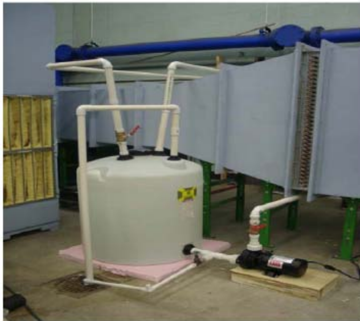
Figure 12. External view of heat exchanger, pump, and tank [33].
