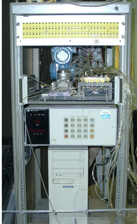
Figure 40. Stand containing the computer, HP unit, transducers, solenoids, and thermocouple jack panel.
