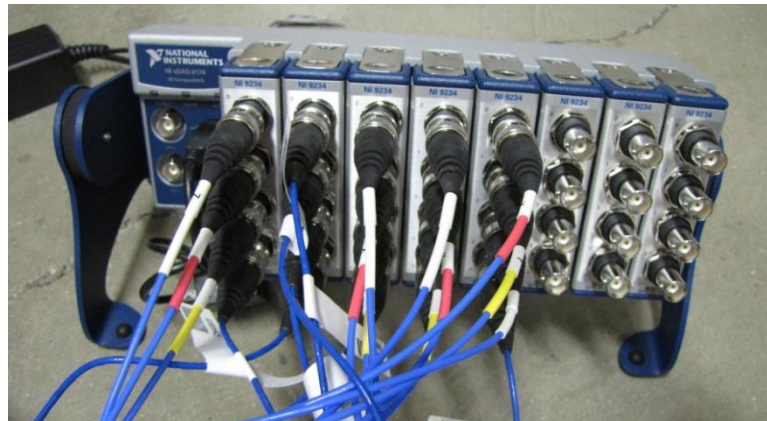
Figure 11. National Instruments cDAQ-9178 data acquisition board used for the testing
