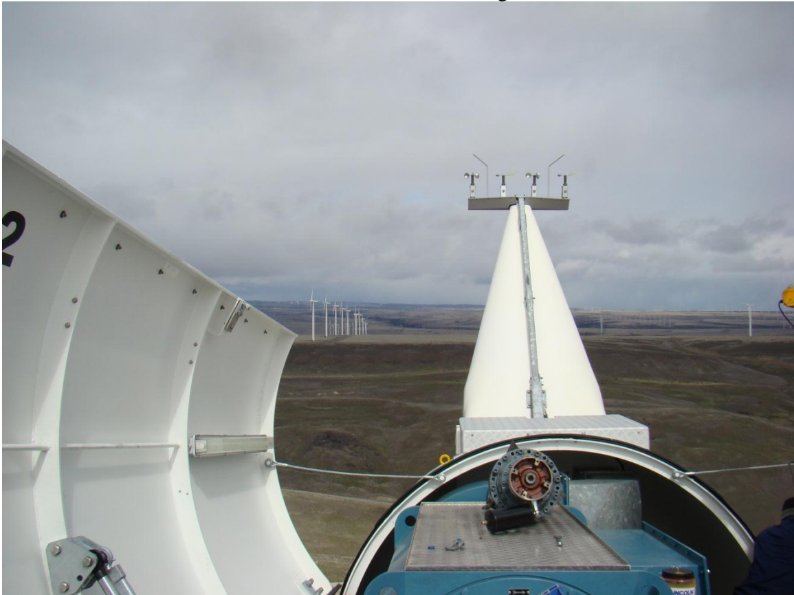
80 meter Siemens 2.3 megawatt wind turbine, White Creek Wind Farm, Roosevelt WA. 2009. Personal photograph by Author. JPEG.
