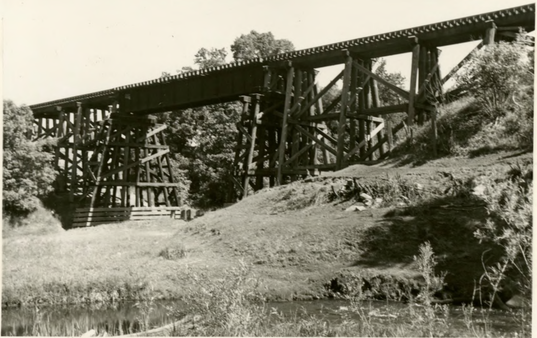
Fig. 14. Railroad bridge crossing the Sand Hill River. The embankment on the far right of the picture was one anchor of the dam used to power the old flour mill.
