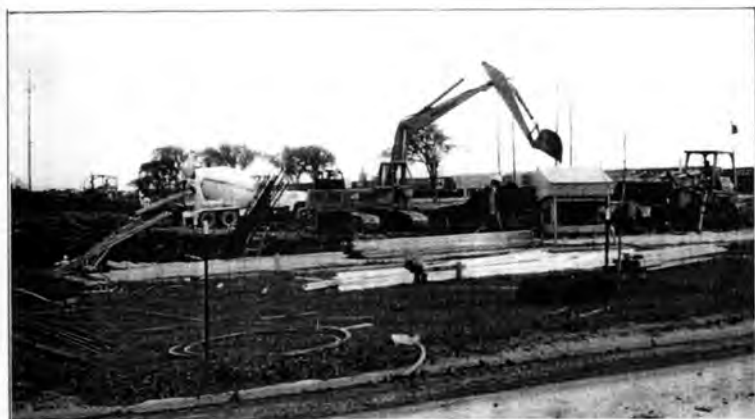
In June 1978, the six tennis courts were removed and a larger shovel than the ceremonial one was excavating the site for the future basement.
