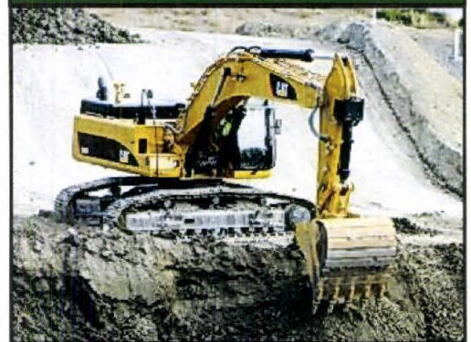
A Caterpillar 345D, the machine selected for excavation in the contaminated region in downtown Mandan. This machine will excavate, load and backfill the downtown site. Trucks loaded by this machine will transport contaminated material to the remediation site, and transport fill material back.
