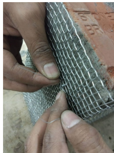
(j) Nailing to fix the wire mesh cage with the 1 st layer of plastering
