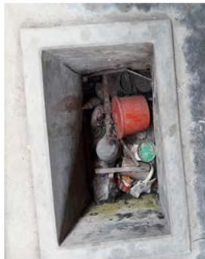
Figure 6: Lack of meter maintenance
