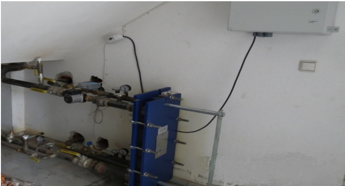
Figure 4: Under building control point
