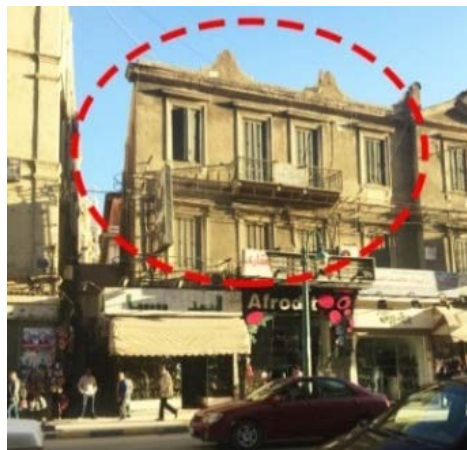
Figure 17: Shows lack in maintenance of buildings façade .
