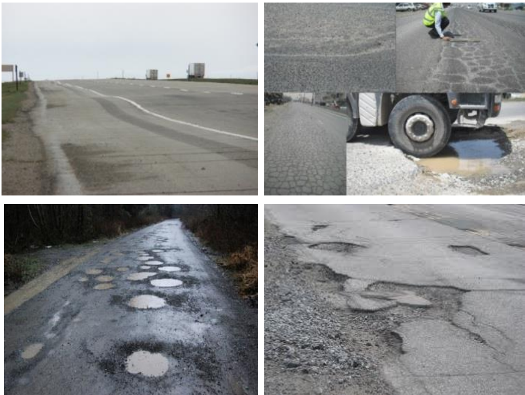
Figure 1-1: Examples of road defects
