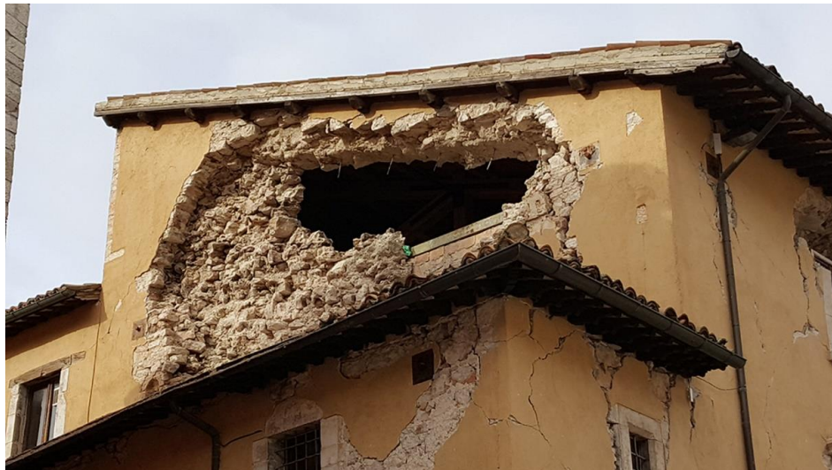
Figure 3. Out of plane collapse of a multi-leaf masonry wall (2016 Amatrice-Norcia earthquake).
