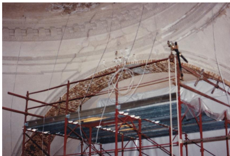
Figure 8. The cracks of the triumphal arch of the main nave.
