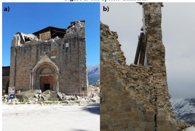
Figure 2. Collapse of the St. Agostino church in Amatrice (2016 earthquake): a) out of plane of the façade after the first seismic shock, which highlights the opening of a sub-vertical crack previously strengthened by cement injections after the 1979 Valnerina earthquake; b) opening and collapse of the failure in which it is possible to see the signs of previous cement injections.
