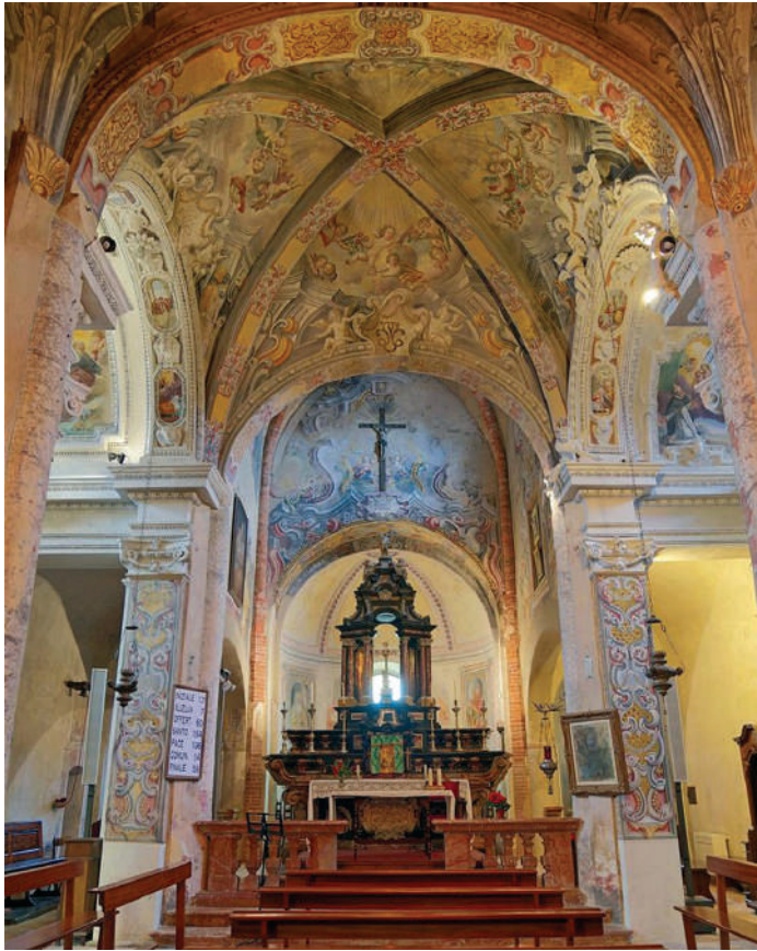
Fig. 4. Dulzago (Novara) Church of San Giulio. Second central aisle covered by a ribbed vault with rectangular ribs.
