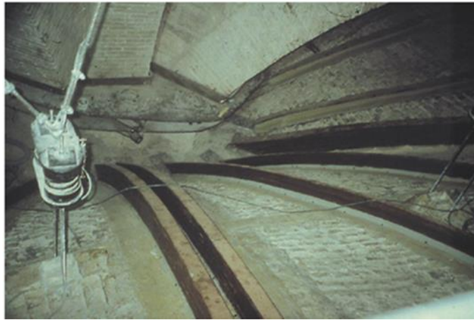
Figure 33: the new ribs, made of a central timber nucleus and external aramid fibres. In the background, the steel belt to anchor the base of the arches which sustain the roof is visible. Source (Croci, 2000).
