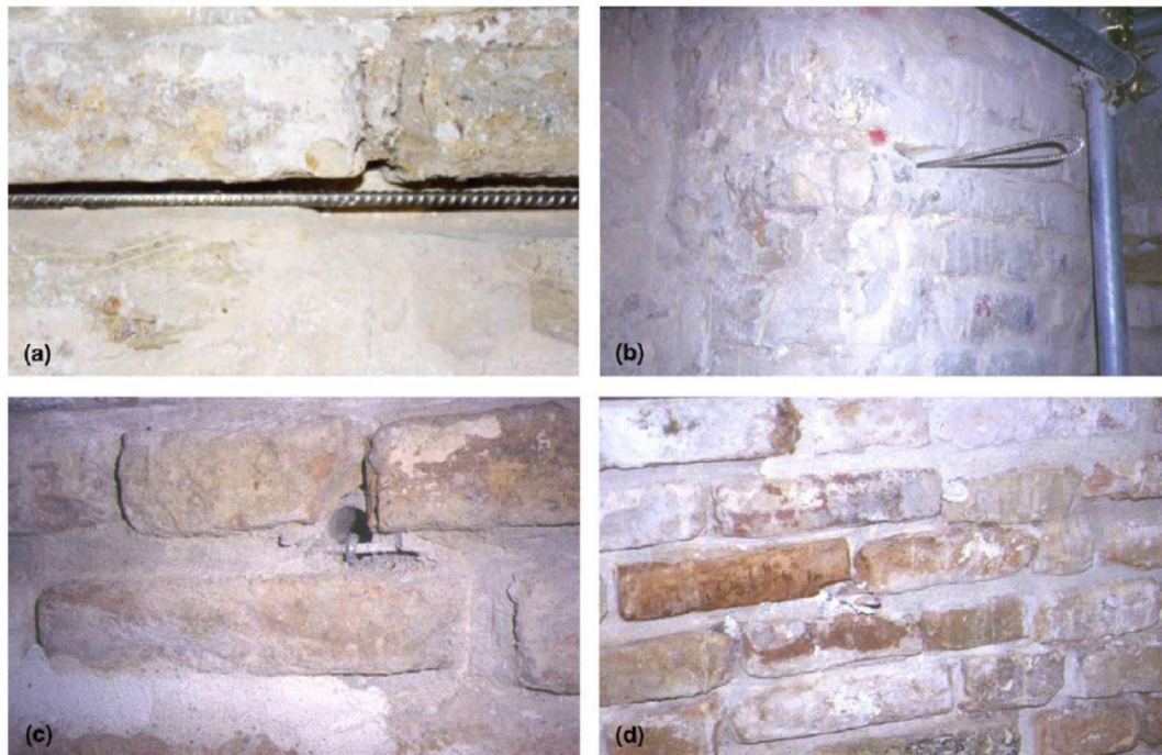
Figure 18: repointing technique , phases of intervention: placing of the rebars (a) and of the anchors (b); view of a joints after repointing (before the injection of the pins' holes) (c); final view (d). Source (Valluzzi, et al., 2005).
