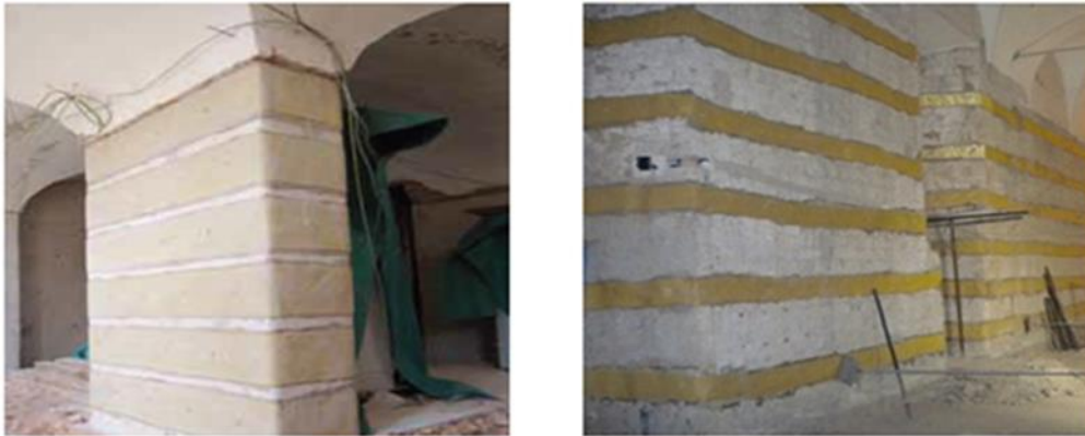
Figure 35: strengthening intervention with FRP in Villa Reale in Monza (sx), and Real Albergo dei Poveri a Napoli (dx). Source (Olympus, 2016) and (ResinProget, 2012).
