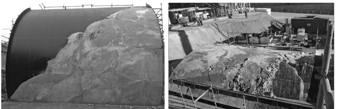
Fig. 5. Test site developed before the starting of the excavation in Brisbane (photos Mapei's archive).
