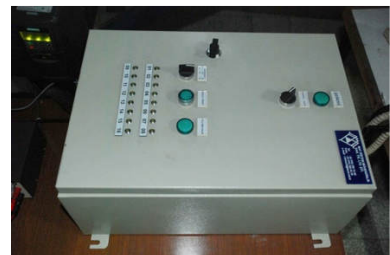
Figure A.12: Valves control unit.
