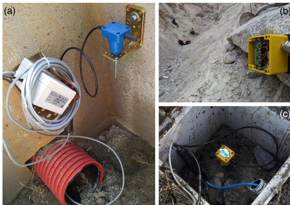
Figure 4 - Different methods of installation of the geophones: (a) embedded in a concrete manhole, picture taken in the Gatria basin (Northeastern Alps, Italy); (b) fixed on rock, Chalk Cliff monitoring station (Colorado, USA); (c) directly dug in the ground, Marderello catchment (Northwestern Alps, Italy).
