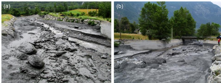
Figure 29 - Detail of the Malo torrent channel bed the day after the debris flow: (a) deposits in the channel bed, photo taken from downstream to upstream; (b) deposits in the channel bed and traces of the passage of the flow on the bridge abutments, view from upstream to downstream (photos taken in the same location where the frames presented in Figure 28 were shot).
