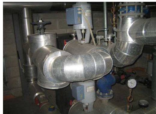
Figure – motorised valves
