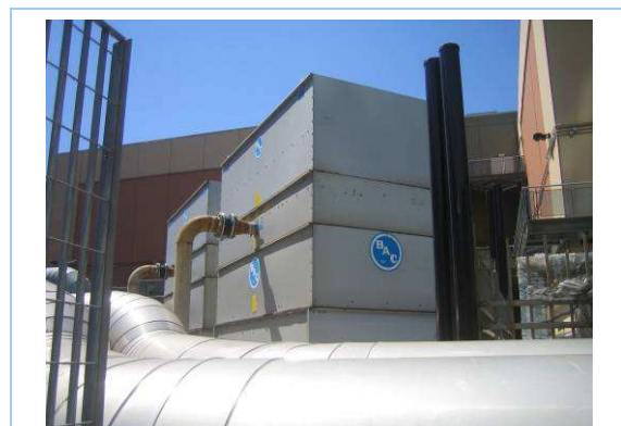
Figure – evaporative towers
