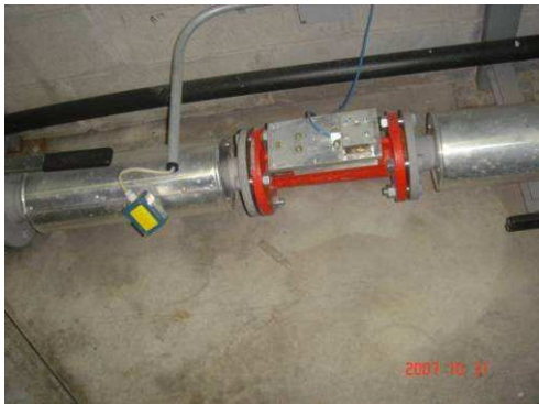
Figure – Heating consumption meter
