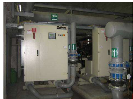
Figure – Cold generator Plant
