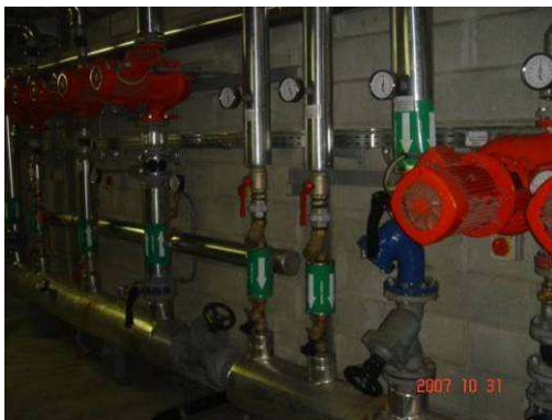
Figure – Pumping system
