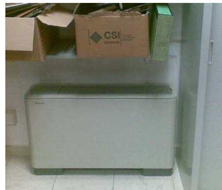
Figure – Internal unit in a inefficient position
