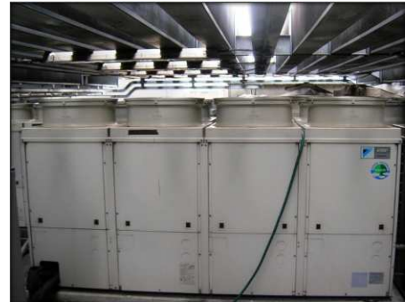
Figure – External units
