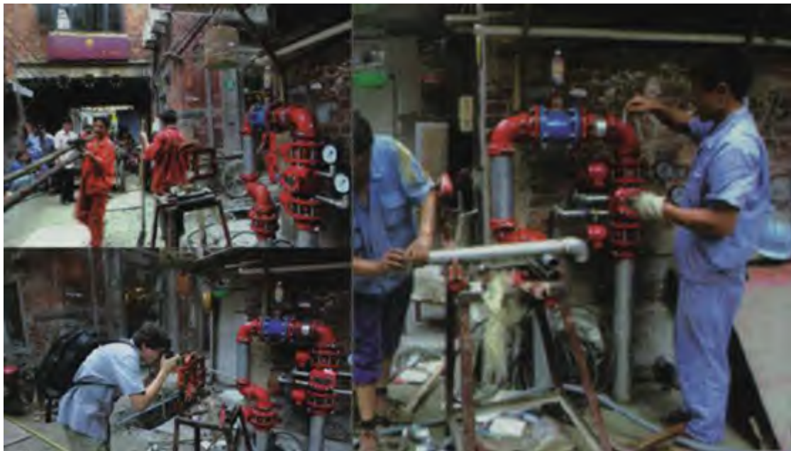
Figure 5-29 The renovation of fire control facilities ,2008 (Source: KE Xiongbin and others, “The Protection of Characteristic Streets in Modern City:A Case Study of Shanghai Tianzifang,” HUAZHONG ARCHITECTURE, 2011, 184–188.)
