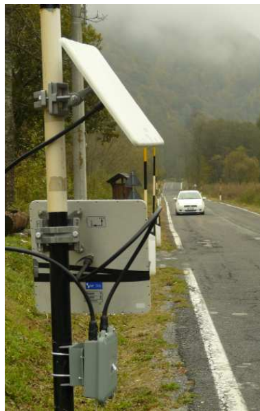
Figure 3.4: Antenna configuration at the RSU: antenna link with CC at the top, and with the OBU at the bottom.
