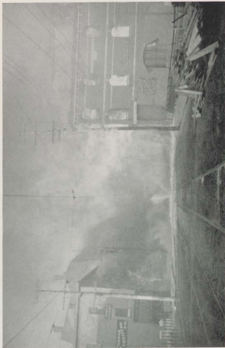
Demolition of the Bangor Savings Bank building in the great conflagration of April 30, 1911
