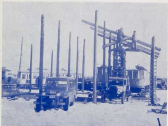
Carhouse construction is one of the many types of activity from which volunteer workers gain valuable field experience.
