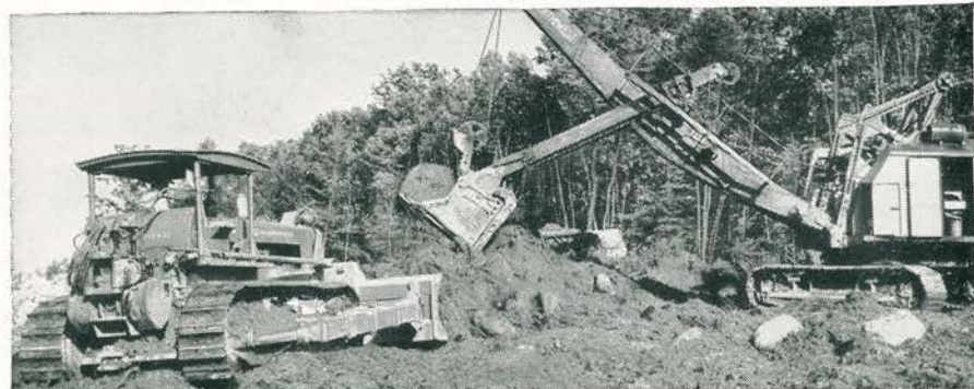
PACIN' THE BIG DIPPERS. Latrobe Road Construction Co., Inc., Latrobe, Penn., uses three TD-24s on its subcontract with Savin and Supt. F. E. Crowell states, "The TD-24 is the only crawler, bar none, that's been able to keep ahead of our big shovel operations".
