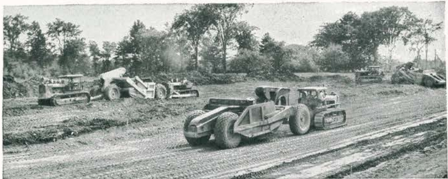
DIGGIN' IN FOR DEMATTEO. "After six weeks of rain it's mighty nice to see our TD-24s delivering 24 cubic yard payloads to help us get back on schedule" reports F. L. Kirby, superintendent for DeMatteo Construction Company, Quincy, Mass. Eight TD-24s are on the job.
