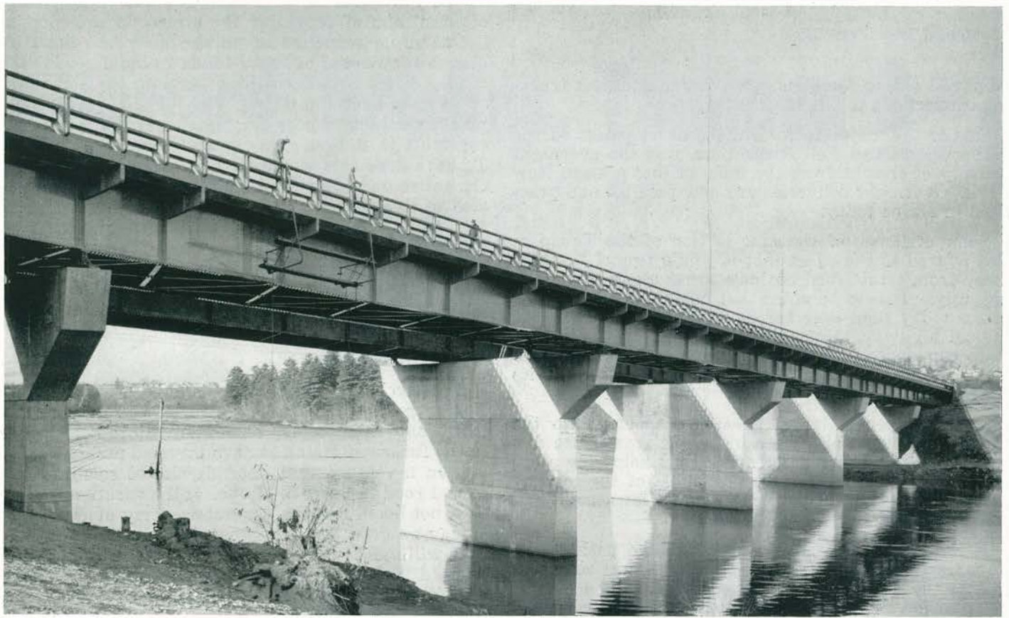
ANDROSCOGGIN RIVER BRIDGE AT LEWISTON, MAINE carrying the Augusta Extension of the Maine Turnpike 6-span continuous plate girder bridge, 845'-8" long
