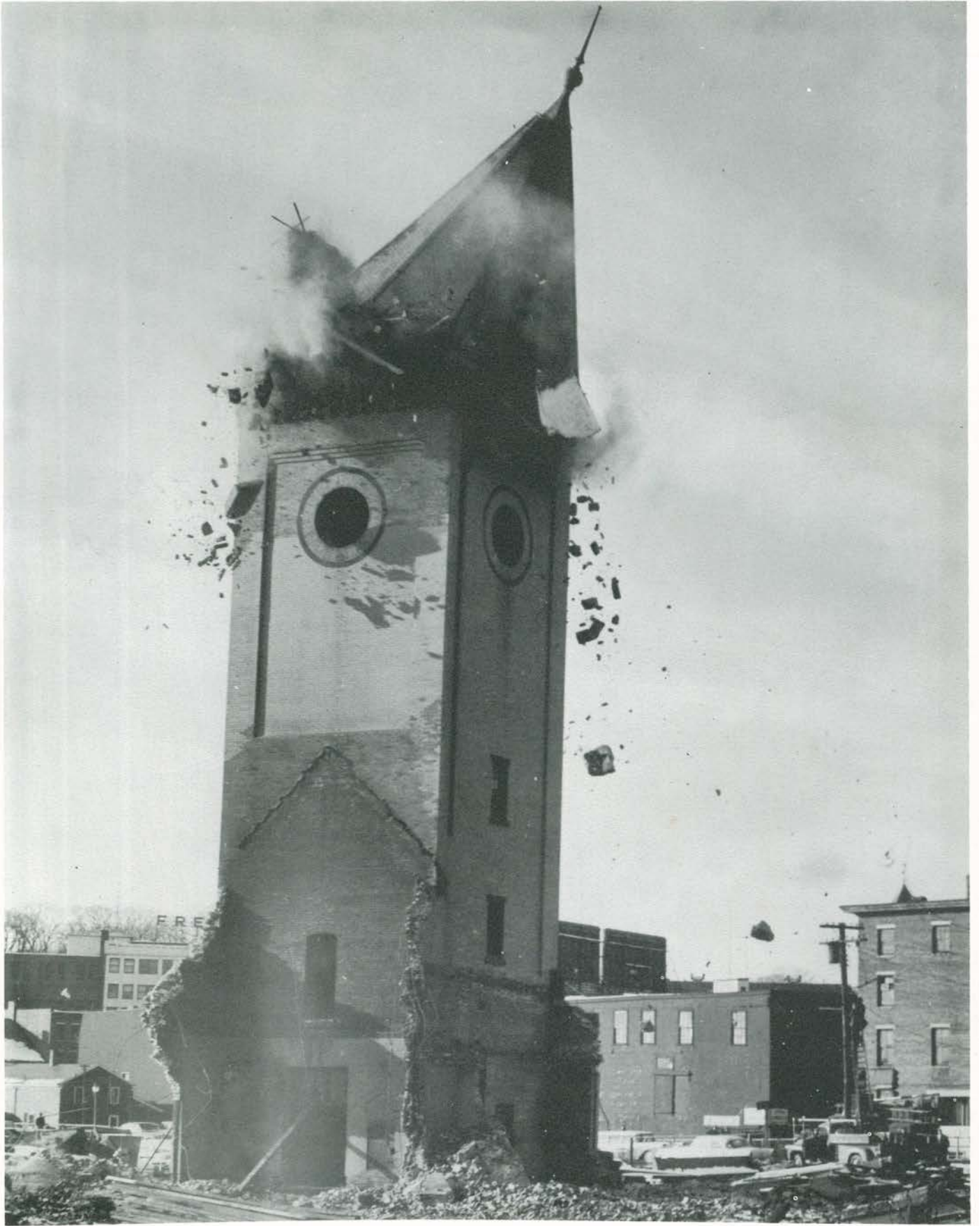
As the old Union Station topples to the ground, an era of Bangor's life is closed forever. A new shopping center is to be erected on the site in the near future.
