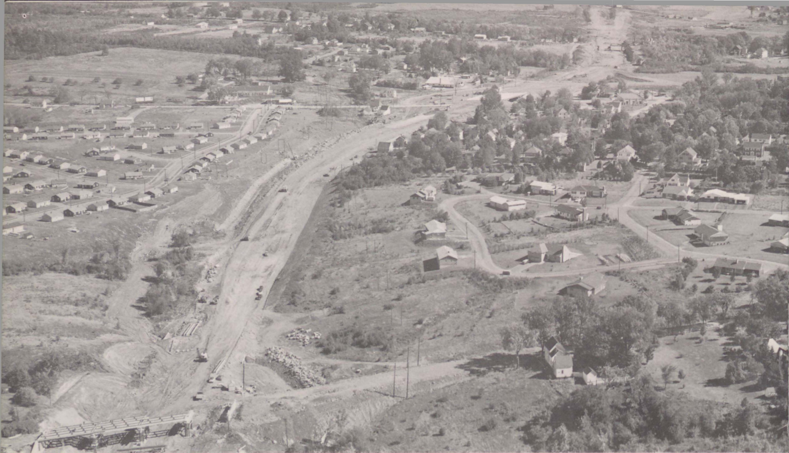
View of Interstate highway construction looking northeasterly. Kenduskeag Avenue overpass is in left foreground. Moving toward top of picture expressway will be carried over Broadway, then under Essex Street; at very top is Stillwater Avenue overpass.
