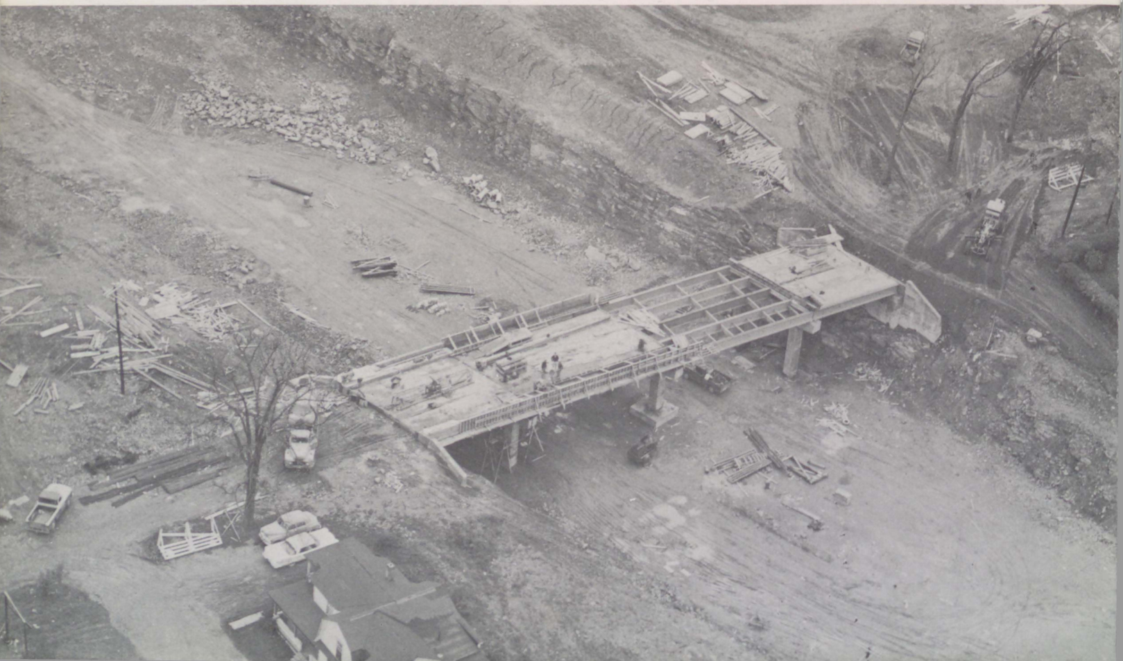
This four-span structure will carry Essex Street over the Interstate highway. Steel beams are in place and construction crews are placing the reinforced concrete deck. At this point and near Kenduskeag Stream men excavated huge quantities of rock.
