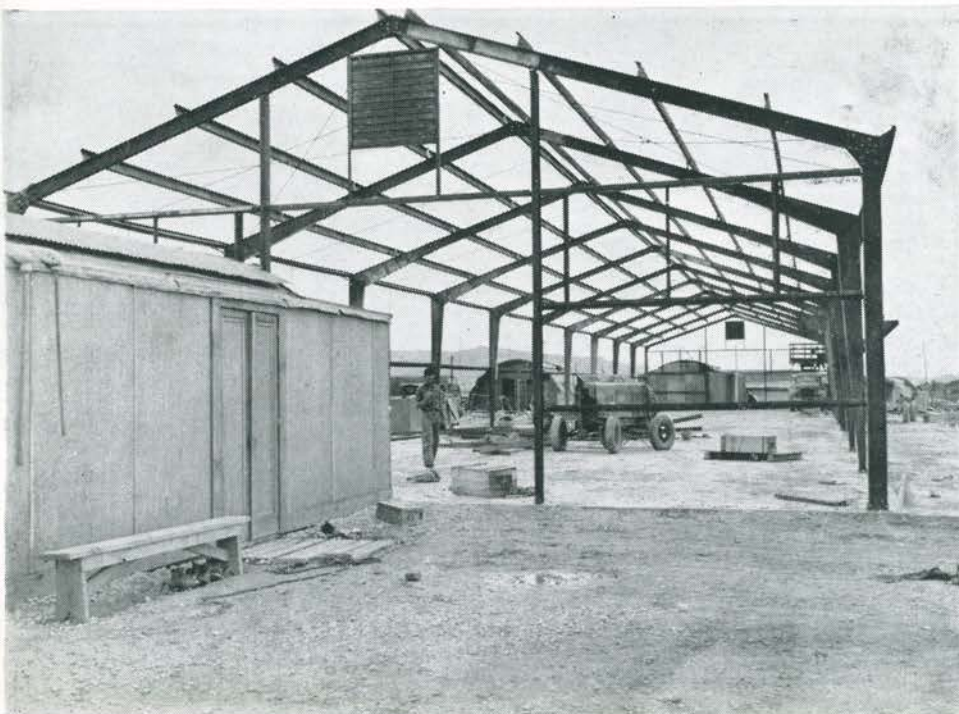
Pictured here is a new type of steel frame construction the 145th used to replace the terminal building at Yonabaru.
