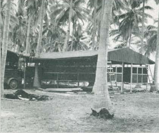
Group S-2, the War Room, and S-3 in the process of construction.
