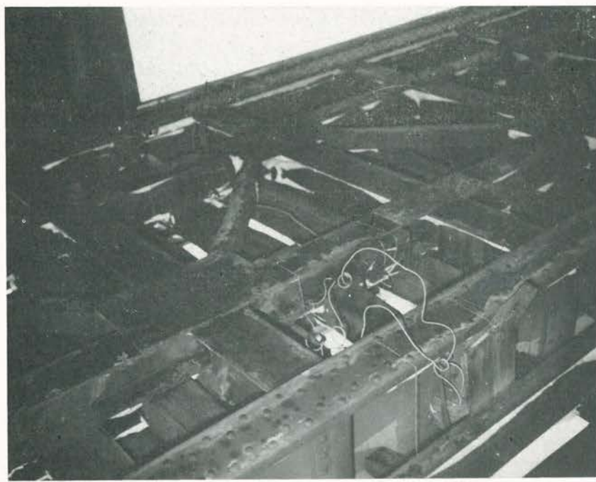
Railroad bridge prepared for demolition in defense plan. Picture shows detail wiring of charges
