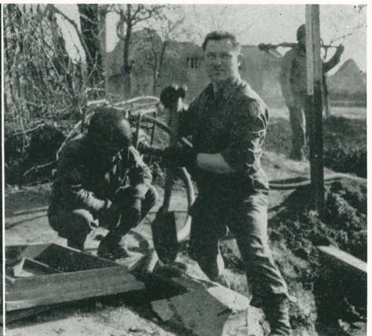
Sgt. Webber and Cpl. Jaycox checking a German city water main before setting up water supply point
