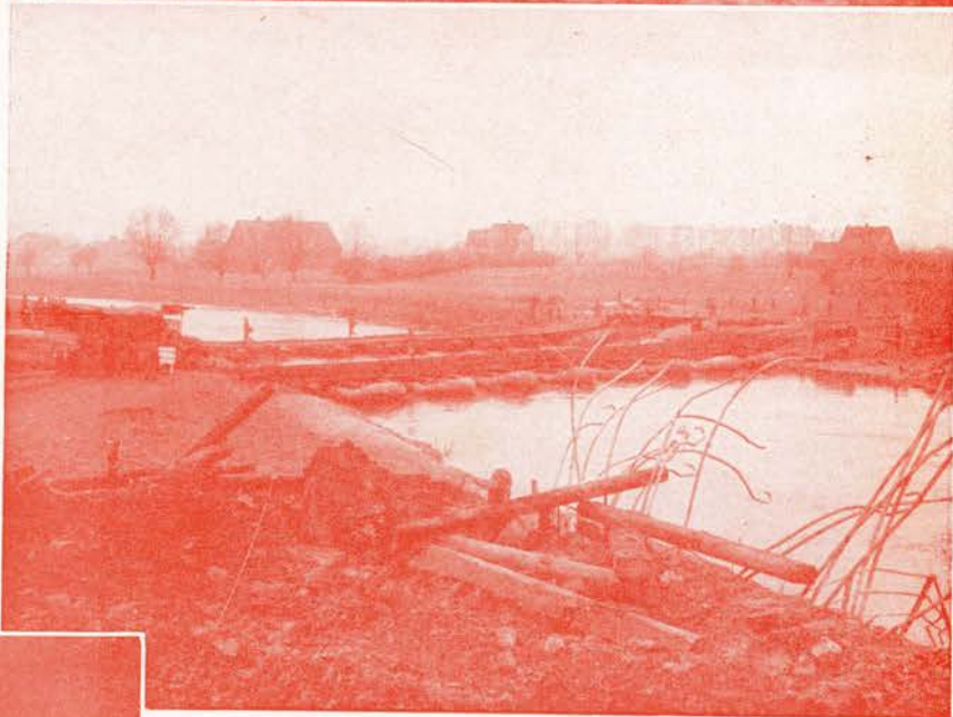
Floating treadway and pon- toon bridges constructed by Company C across Lippe River
