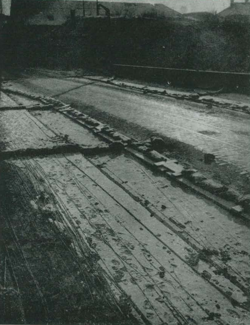
During Battle of Bulge the bridge across Saar River at Saarlautern, Germany, was prepared for demolition by 320th Engineers. Demolition wires protected by planking and sandbags. January, 1945
