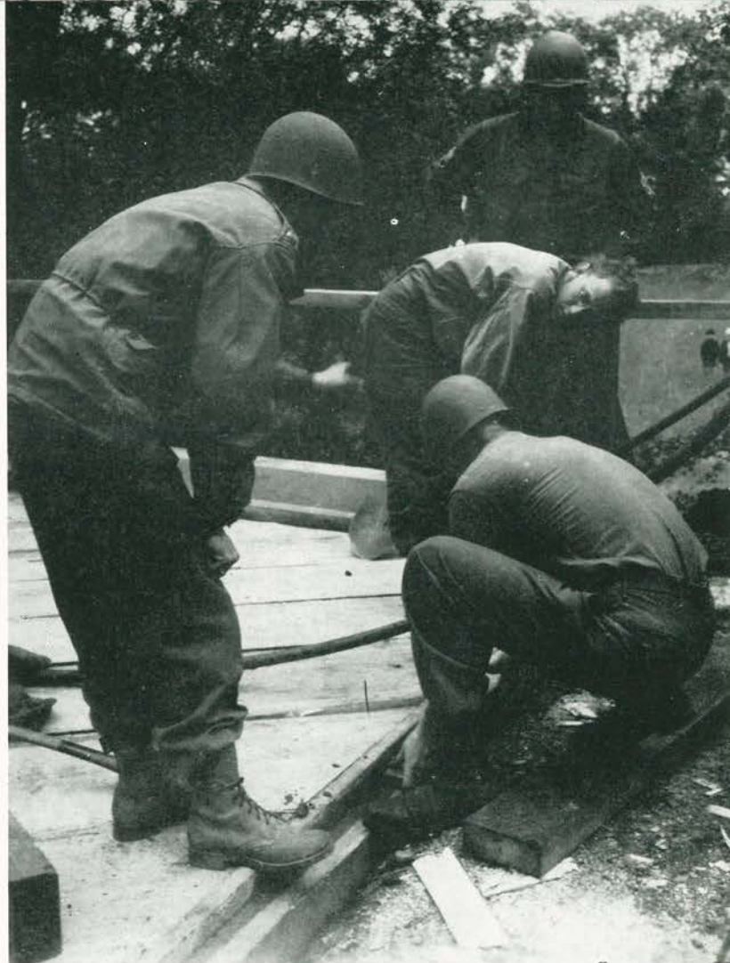
Company C constructing wooden trestle bridge across small stream Lieutenant Keough supervising details of construction
