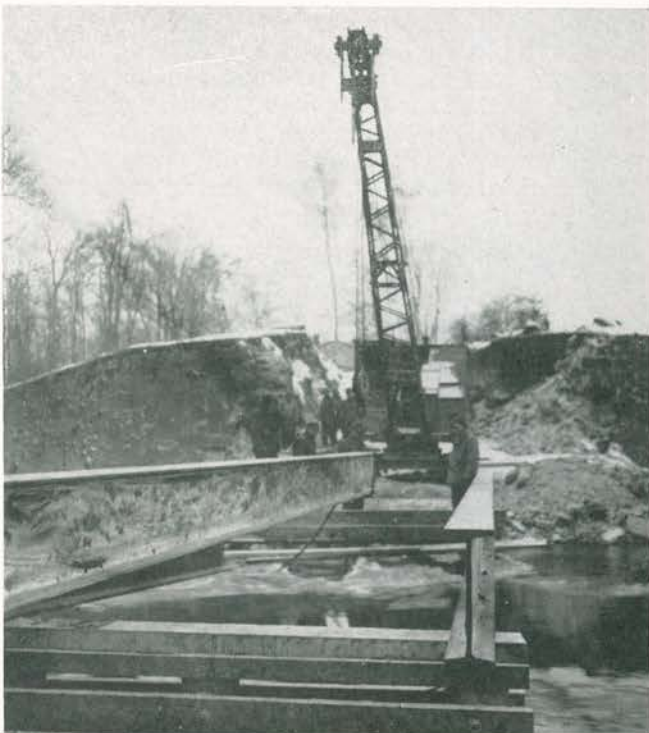
Placing steel stringers in place during the construction of a fixed bridge across the Saar River
