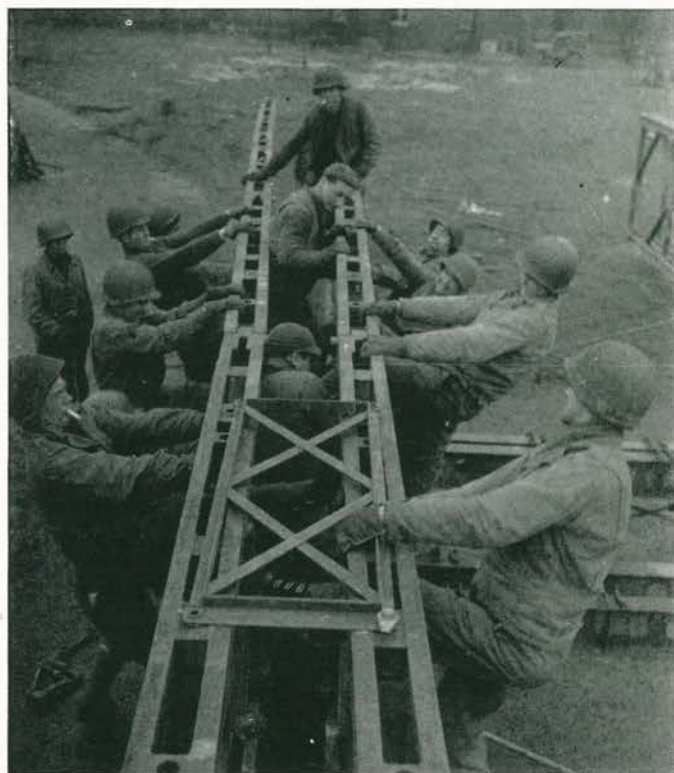
Double Double Bailey bridge being launched by Company A at Wanssum, Holland
