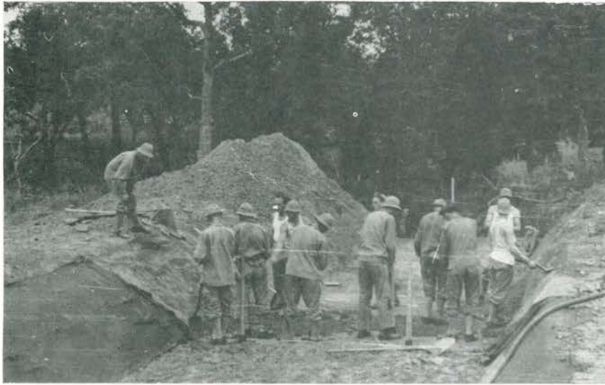
Camp Swift, Texas. 320th Engineers constructing spillway to dam using soil cement materials for surfacing of sides and bottom of spillway.
